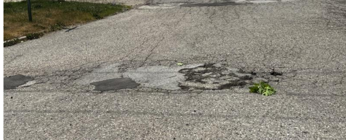
Poorly paved roadway along Union Street.
